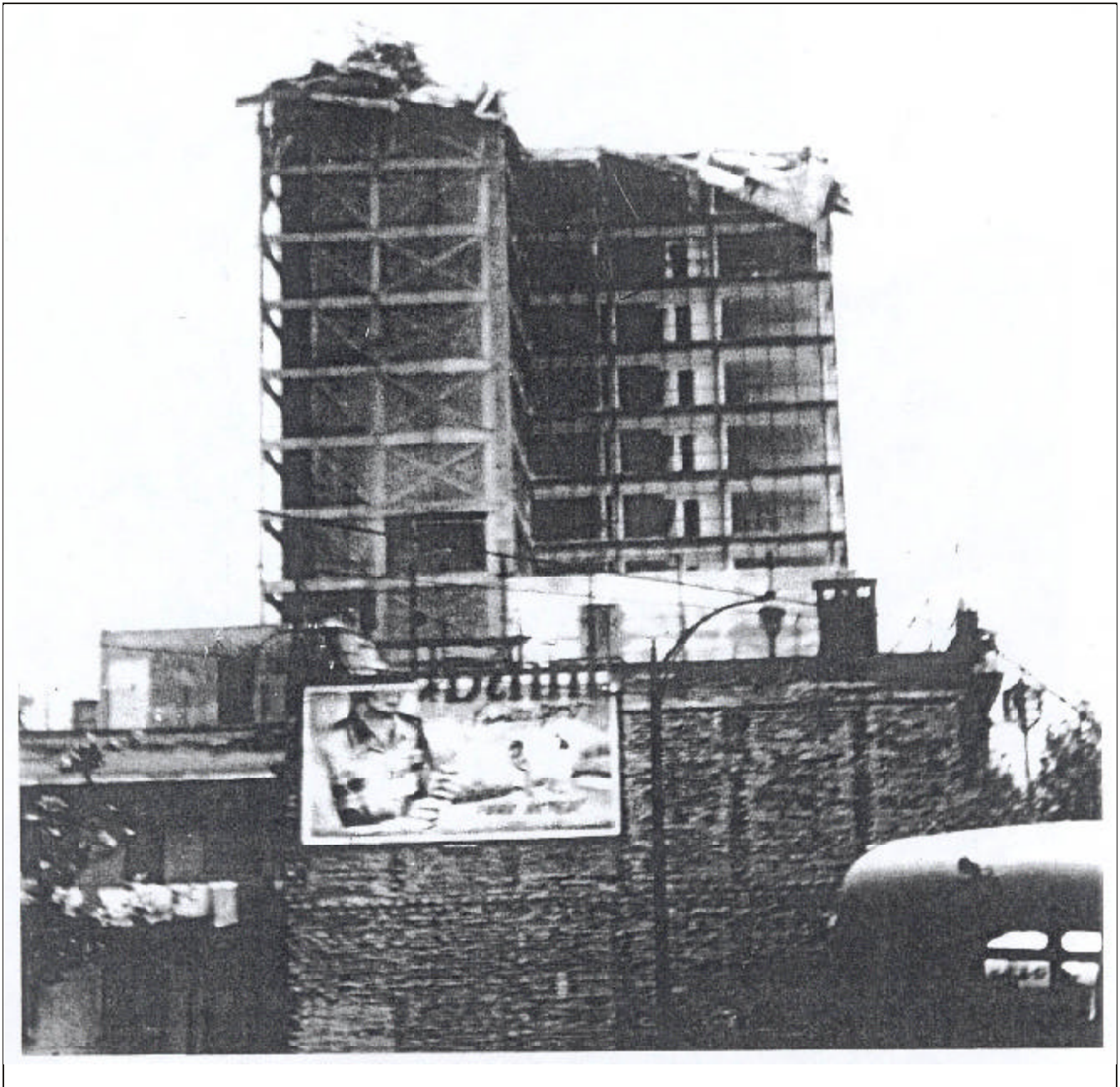
Photo 2. "Whipping effect" in the upper floors because of seismic action
