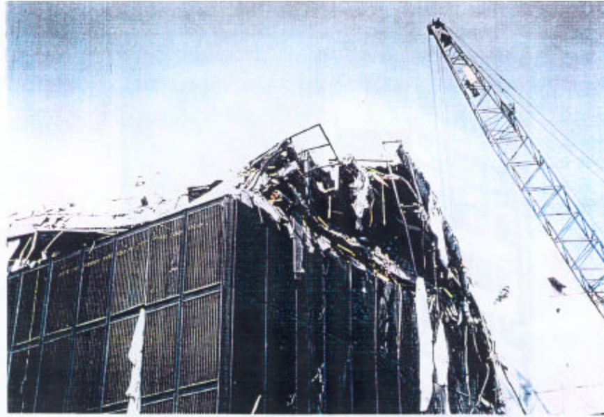
Photo 4. "Whip ping effect" in the upper floors because of seismic action
