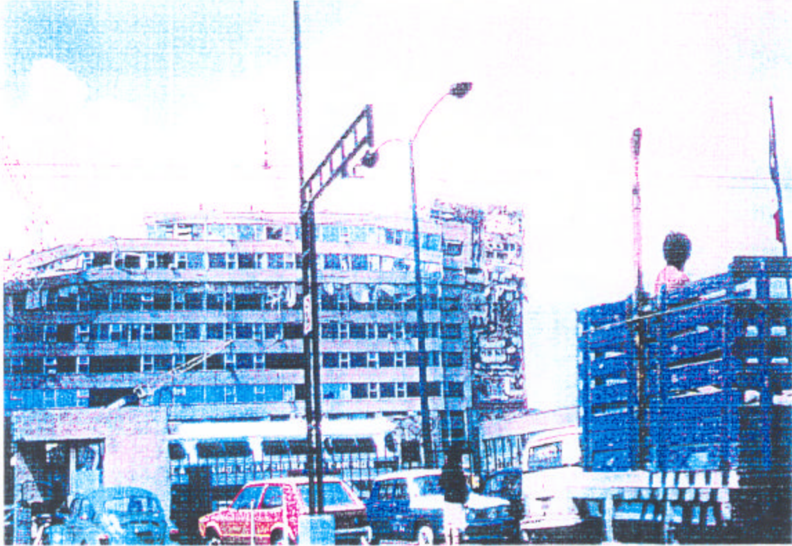
Photo 6. Failure of head-frames in the upper floors because of seismic "torsional whipping action"
